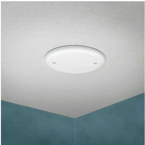
Capped Electrical Ceiling Box
